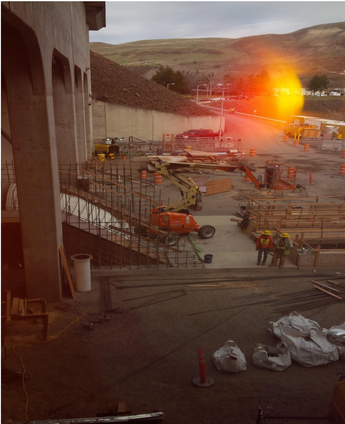
AWS 10' valve room progress. The halo means its close to the end.
